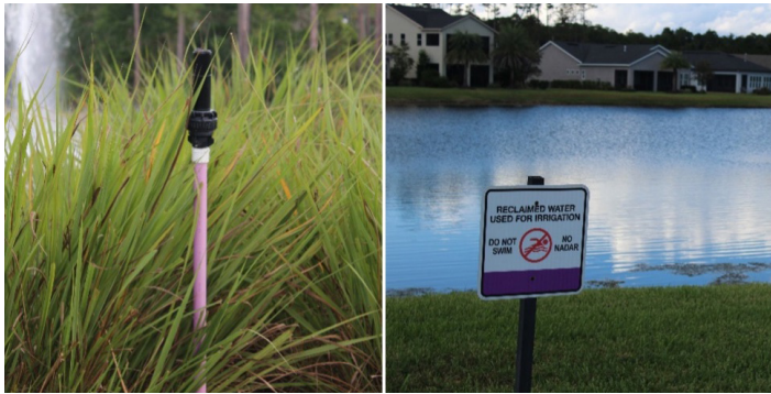
Figure 2. All reclaimed water piping, fixtures, valves, heads, etc. are required to be purple in color and labeled “Do not drink this water.” Credits: Terra Freeman, UF/IFAS
