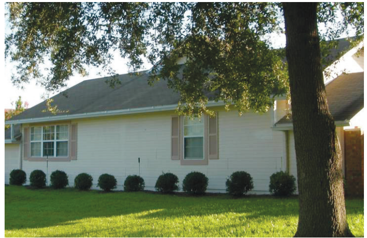
FIGURE 5. Shrubs along wall are overtrimmed.
