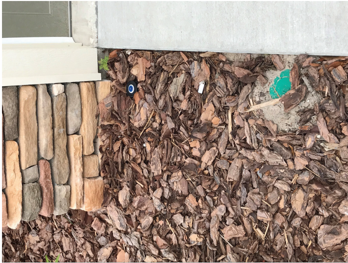
Figure 2. Faux rock is a popular wall covering. Pine bark mulch is covering the inspection space along the concrete slab combined and irrigation installed too close to the wall in violation of the current building code. The Florida building code requires that irrigation be installed 1 foot or more away from a building sidewall. Irrigation that “water walls” is considered a conducive condition that can void termite control warranties. There is enough moisture for weed growth. A termite bait was wisely installed in this area.
